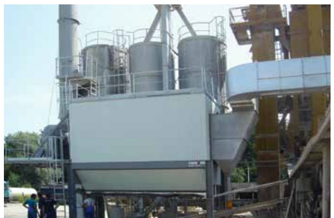
Integrating a new filter into an existing old plant.
