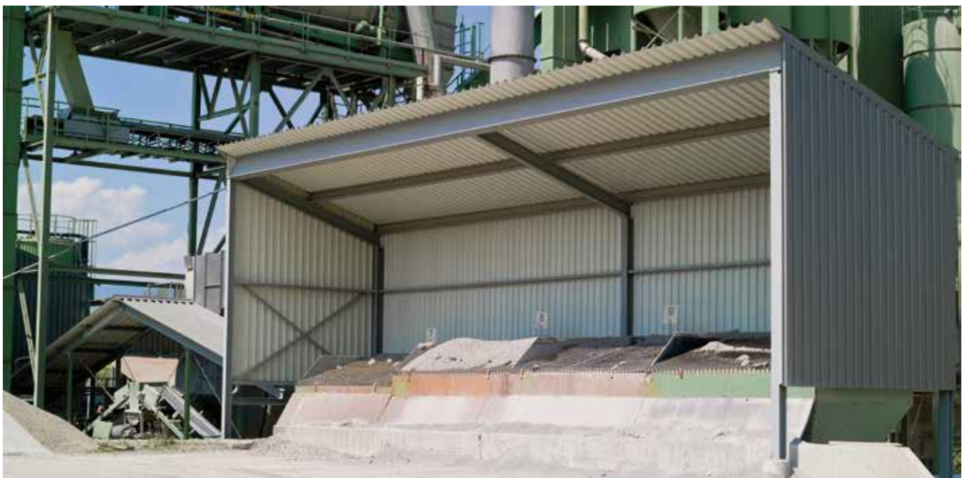
Roofing over the pre-feed for crushed recycling is an efficient way of cutting fuel consumption.
