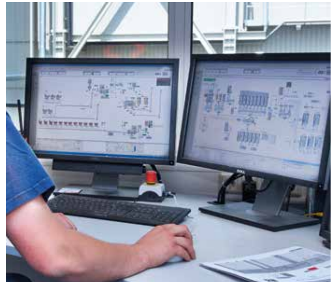
Control station for controlling two asphalt mixing plants.
