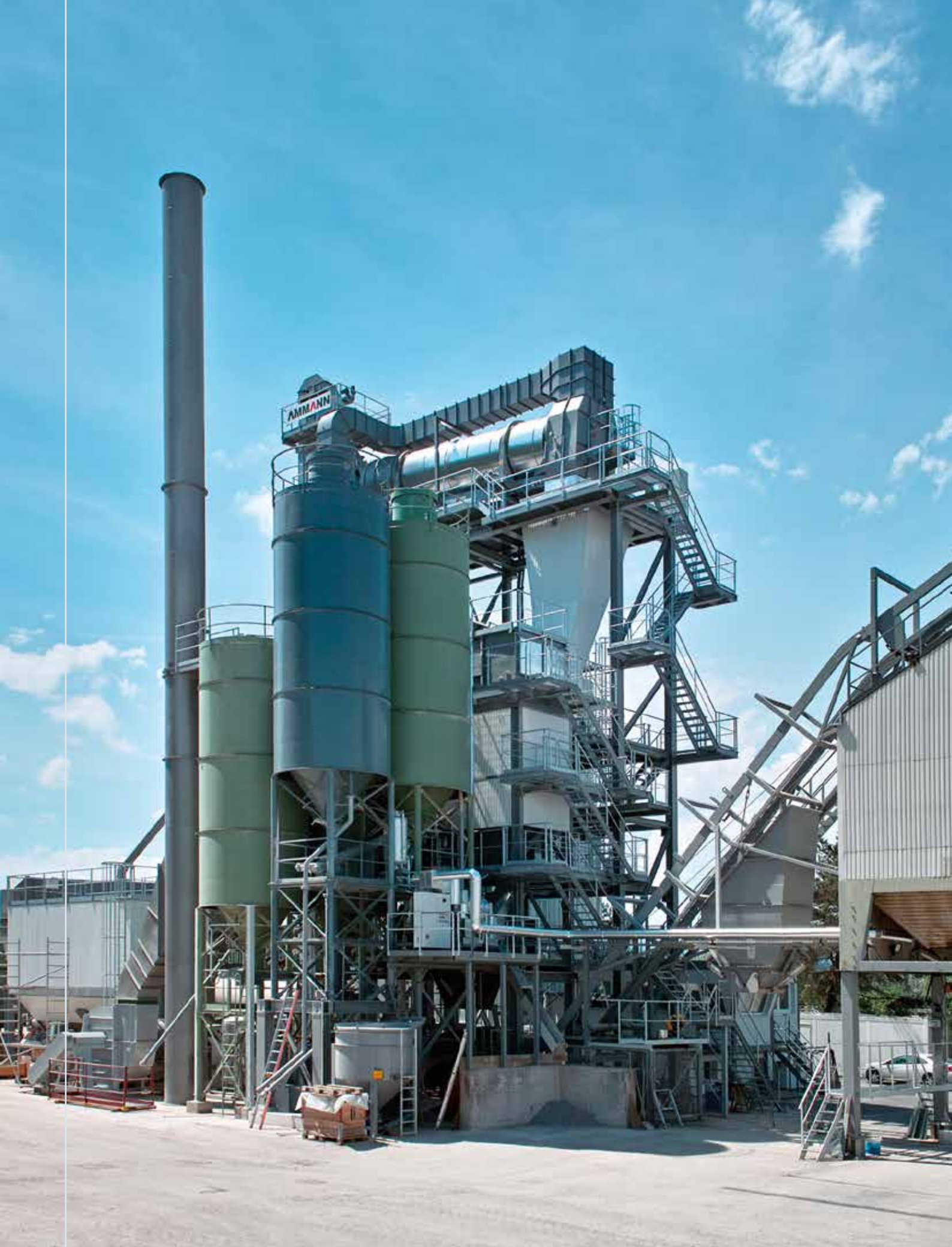
Partially modernised asphalt mixing plant. Newly installed: Control cabin, bitumen tanks, filters, Uniglobe 200 tower.
