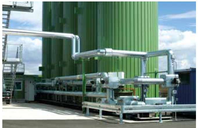
Bitumen plant integrated into the plant control.
