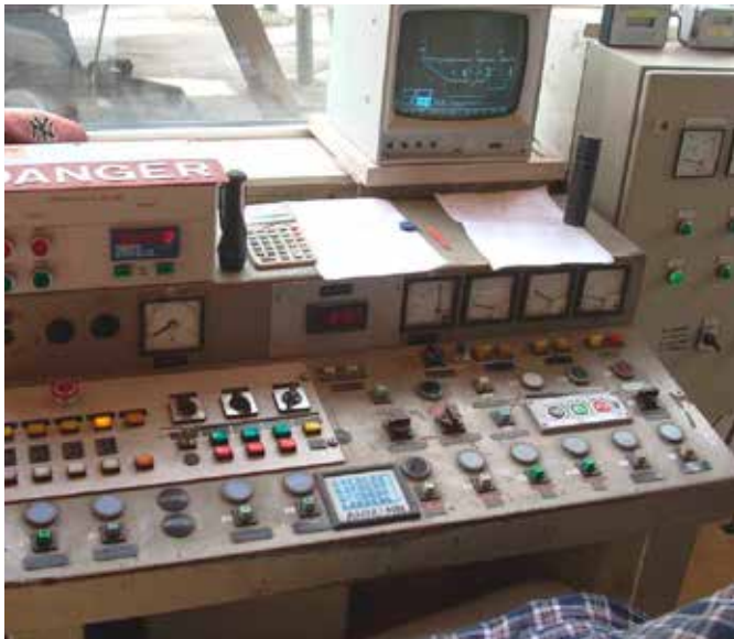
Outdated control technology.
