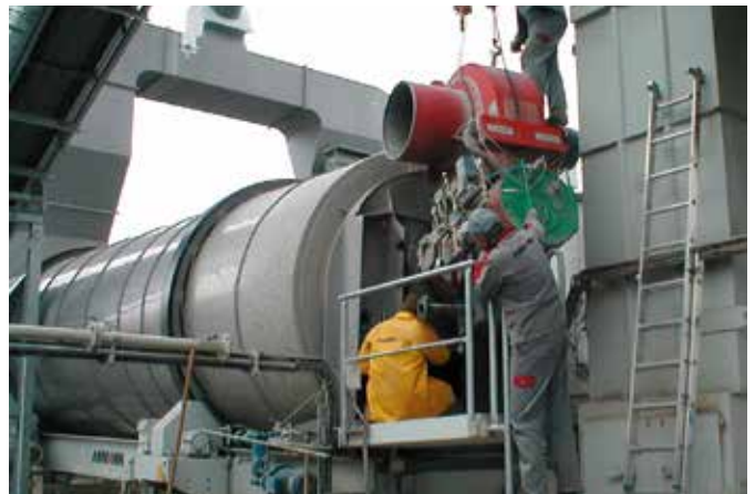
Installation of a TAB burner. TAB stands for Thermal After-Burner. These burners suck off bitumen vapours, for instance in the discharge area beneath the mixed aggregate storage silo, and then burn them in the after-burner.
