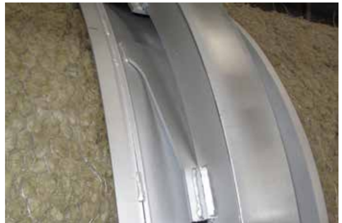
High performance drum insulation beneath an aluminium covering. Precision drum support ring spring mounted to compensate the thermal expansion.
