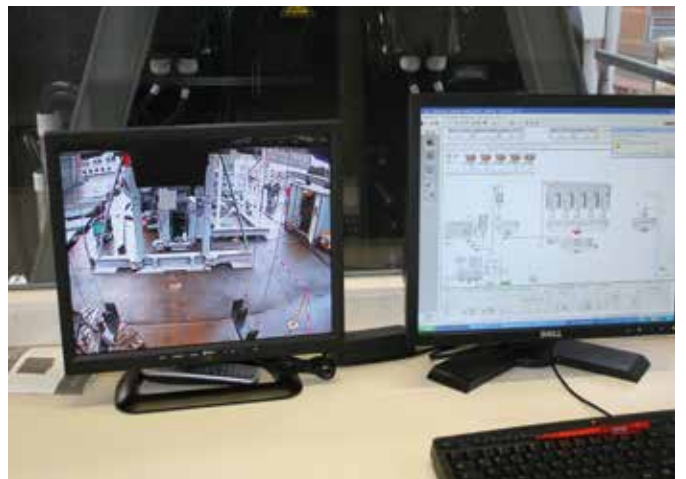
Excellent view of the plant: The command room is located at the height of the mixer. The loading area is monitored with a camera.
